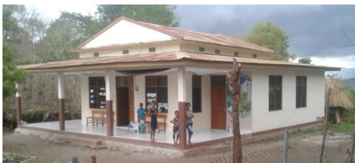
The clinic in need of repairs due to termites.
